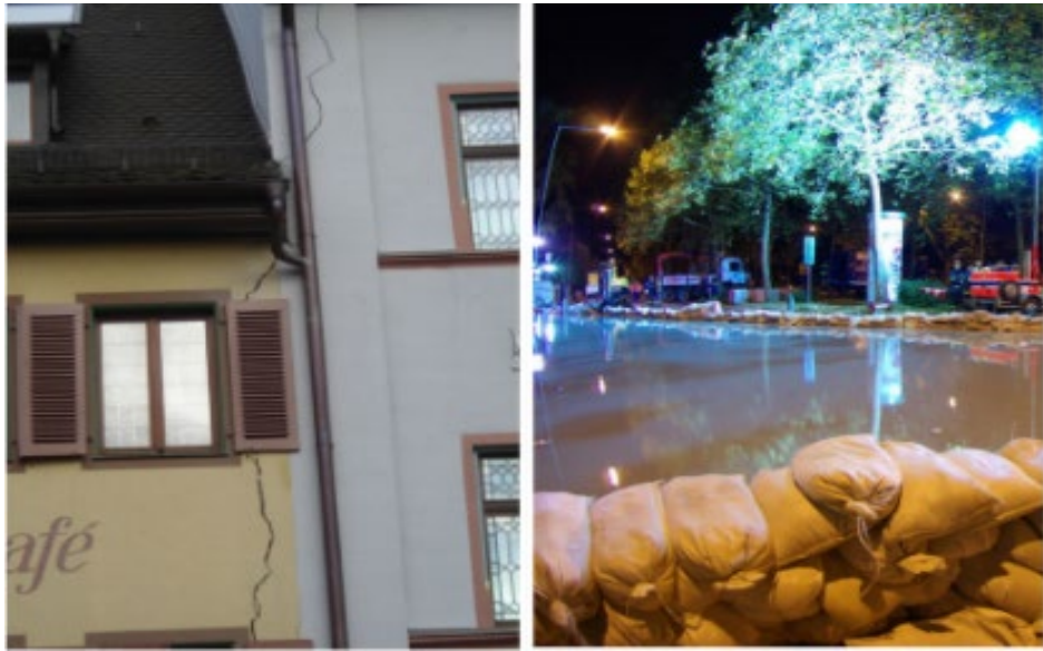
Figure 1: Structural damages that occurred in Staufen, Germany due to ground uplift from borehole drilling [3].
